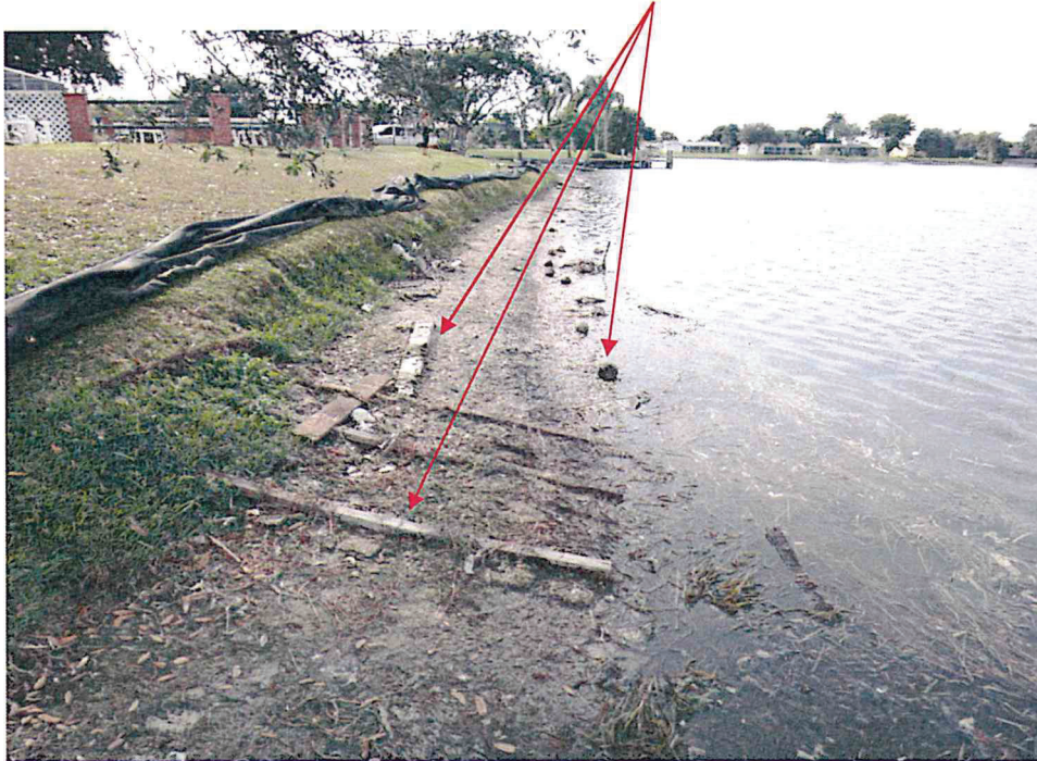
Eroded shoreline to be cleared of debris and larger coral rocks
