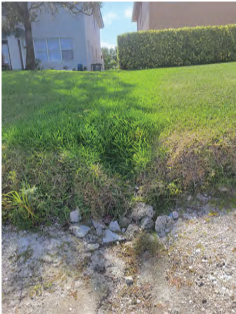
Another erosion area on lake 6 (west bank) between houses
