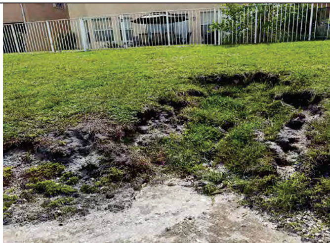
Photo 6: Lake 12 has buried downspout piping
